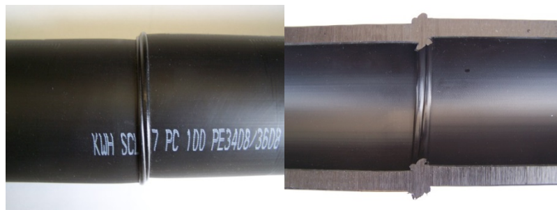
Figure 7 - Pipe misalignment (high-low misalignment)
