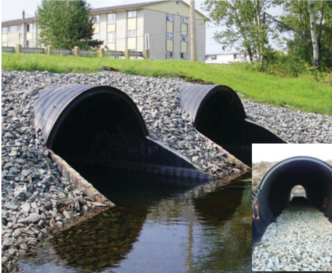
Rocks were placed inside the Weholite culverts to create a natural river bottom
