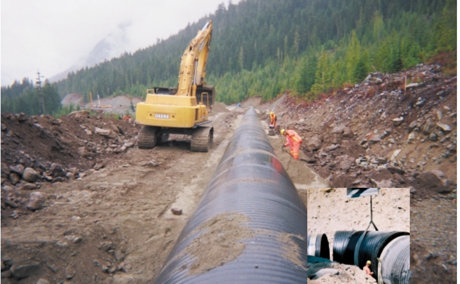
Weholite pipe system carries Rutherford Creek water 3.5 km (1.988 miles) to powerhouse site.
