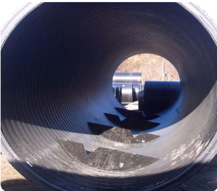
Fish Baffles and Flow Attenuators
