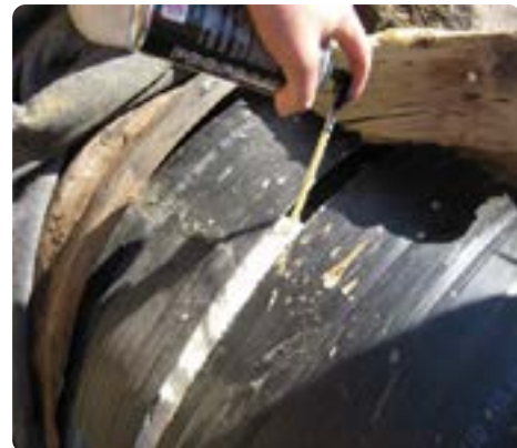
Step 2: Using closed-cell polyurethane spray foam, spray foam in the joint around the entire circumference of the pipe.
